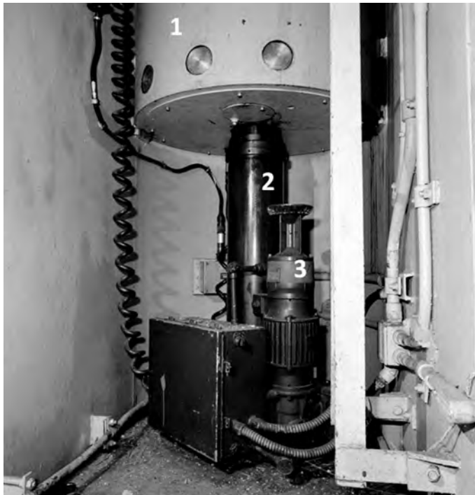
Secondary door fully retracted, Launcher Equipment Room Level 2: 1) 4-inch diameter locking bolts; 2) linear actuator; 3) manual override drive for linear actuator. (Library of Congress)
